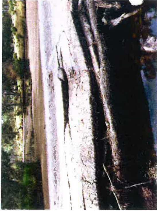
Pre-Construction Photos. The existing causeway was acting as a barrier to fish passage and had totally failed. As a result, it had a load limit of 5T placed on it (Photos & info: Chris Thompson).
