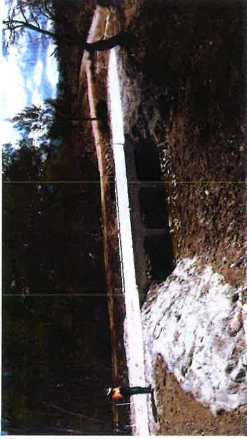
Post Construction prior to Side Track Removal – Note the sedimentation controls in the background and the installation of Box Culverts allowing free fish passage and reinstatement of the natural bed gradient. The stream is currently dry due to the drought. During normal conditions a large permanent pool is located on the upstream side of the causeway.
