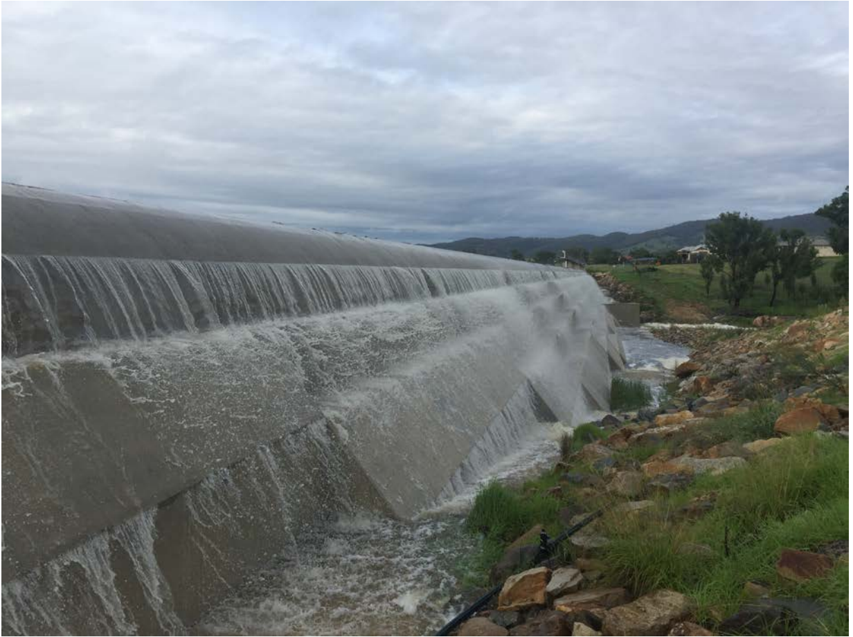
Tenterfield Dam Overtops – Friday, 14 February 2020
