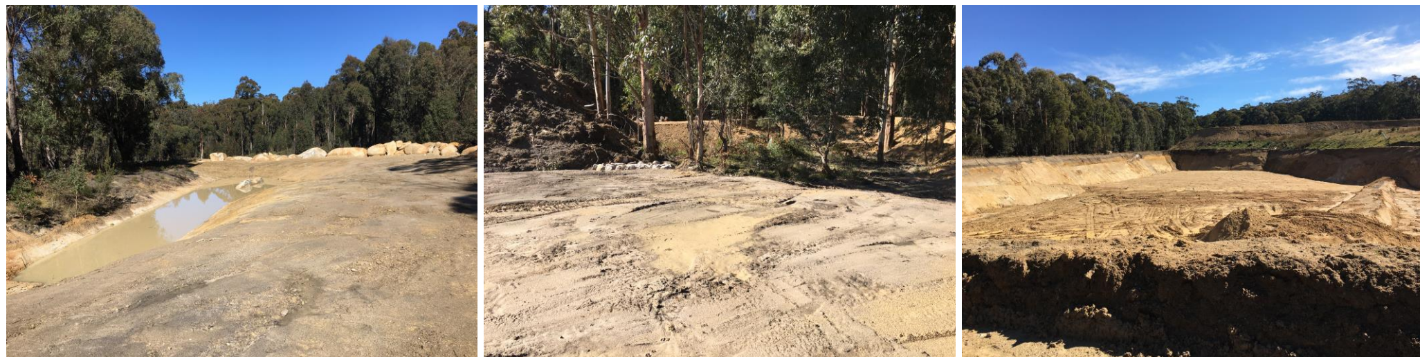
Figure 13, 14 & 15 View south and north side of leachate pond (sediment basin) and view north of cell 5.
