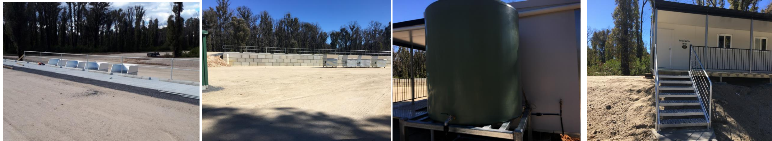
Figure 9, 10, 11 & 12 New wheel stops and handrail installation Water tank installed and Site office stairs.
