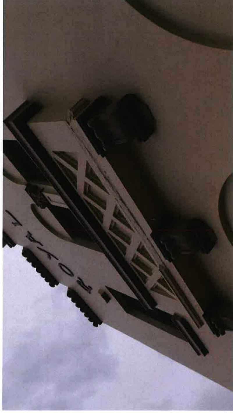
Missing part of moulding. Note new paint scheme (pre approved) in vellum, and olive greens from the interwar examples in Tenterfield.
