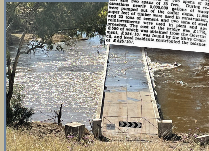
Hynes Bridge on Dumaresq River, during flood
